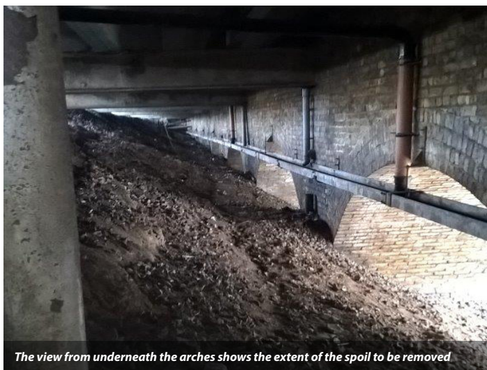
The condition of the arches prior to works. The team carefully removed excess spoil from the embankment to mitigate the risk of subsidence
