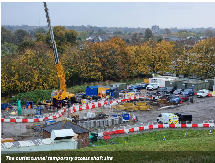
Barhale's site at the inlet tunnel, with the temporary shaft adjacent to the road
