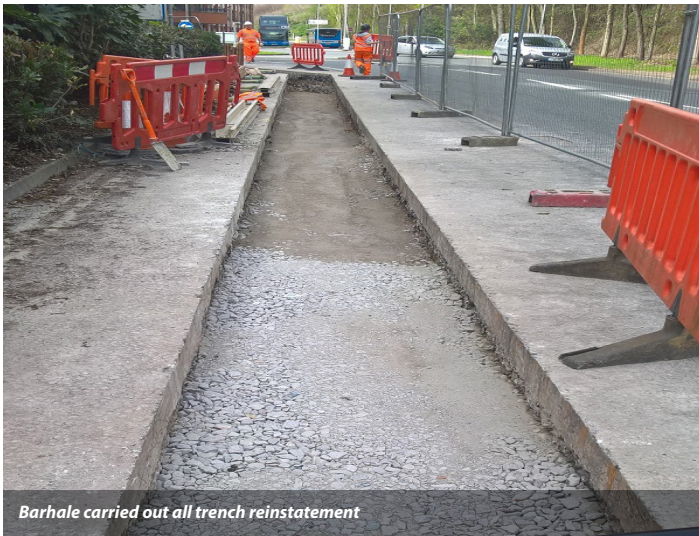
The team excavated 487m of water main trench, 418m of electrical trench and 100m of gas main
