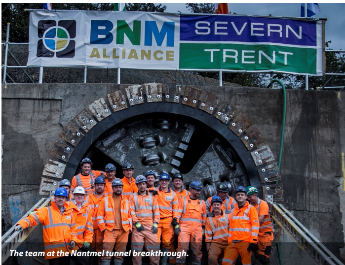
At Nantmel a competition was held at the local primary school to name the TBM. The winning name was Nantmel Supermole.
