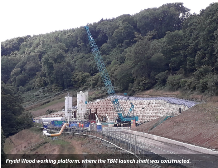
The 45m x 25m secant piled pit (widest point) TBM launch pit at Bleddfa.
