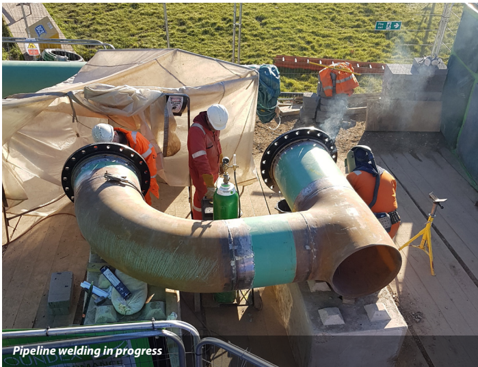
Intermediate Pressure (IP) Gas Main
