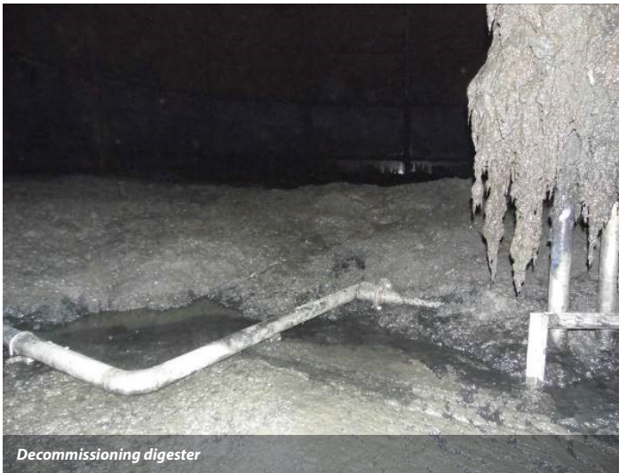
Old gas mixing system
