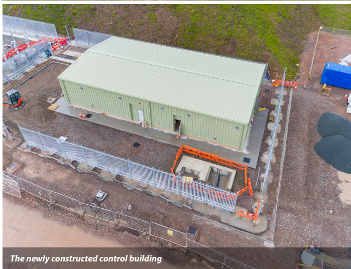
Aerial view of the full site, demonstrating how remote the works were
