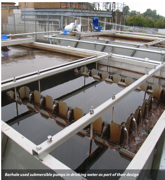
Barhale were responsible for the overall design and construction of the works, taking the concept design from the client and developing the entire (MEICA) detailed design.
