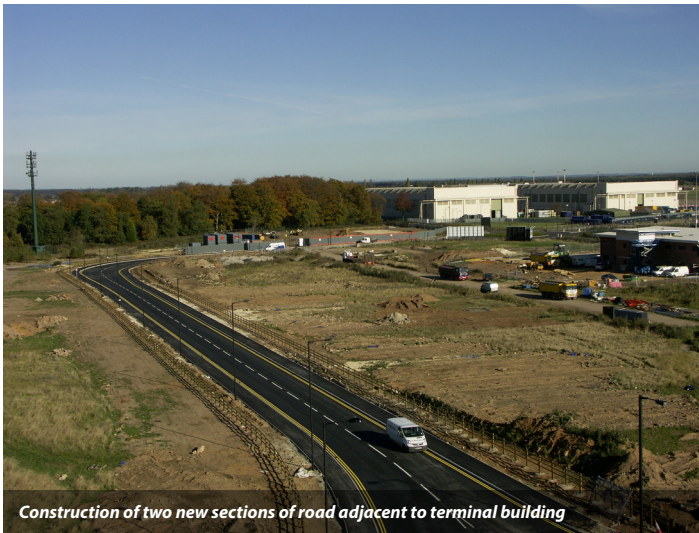
Barhale were contracted to upgrade the existing site infrastructure and services at Robin Hood Airport and Business Park
