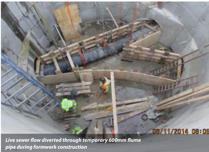
Completed concrete channel to tie together the 3 existing sewer pipes inside the shaft
