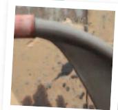
2. The sludge is then pumped into a skip...
