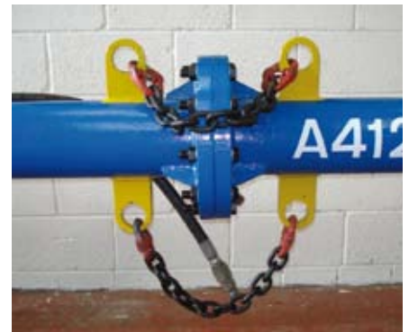
Pole Grab bolts and safety chains
